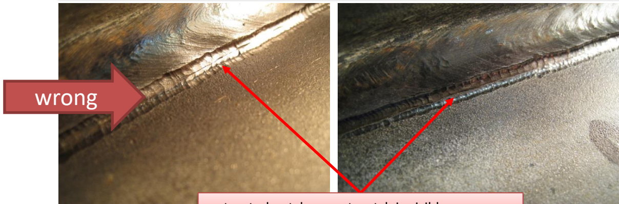
untreated notch => rest-notch is visible
